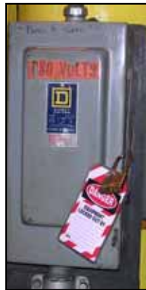
Figure 2-2: Lockout/Tagout on the Power Source Panel
