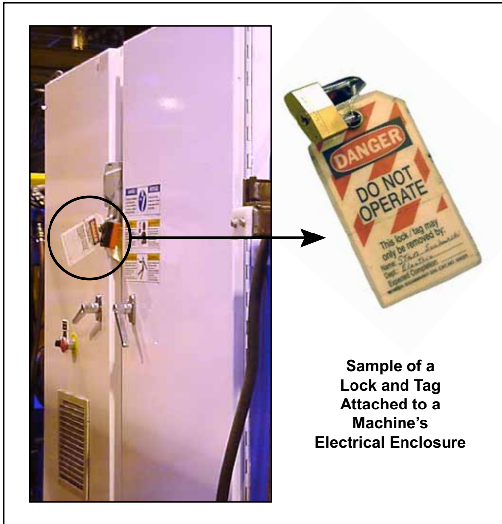
Figure 2-1: Lockout/Tagout on the Main Electrical Enclosure
